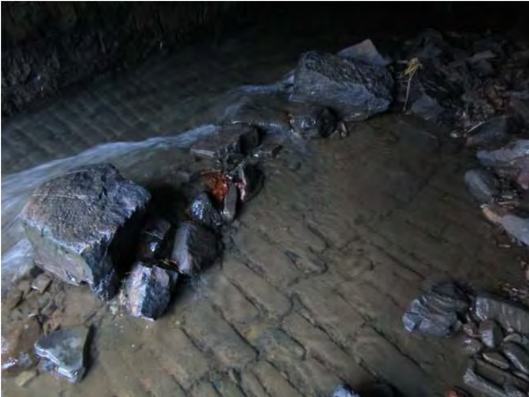
Stream bed within tunnel needing stone removal. Note the lined stone base of channel.. Direction photographer facing: North West
