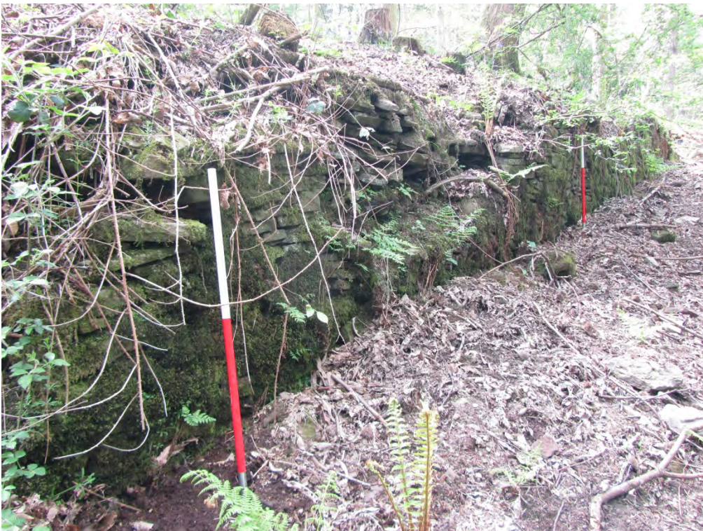
Plate 14: The retaining wall for the track (to the right) between the upper and lower terrace. Photo looking west (Picture; Clive Osborne)
