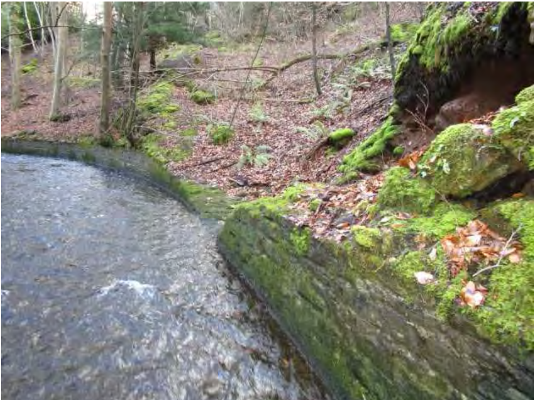
Missing stonework from wall? Direction photographer facing: North East
