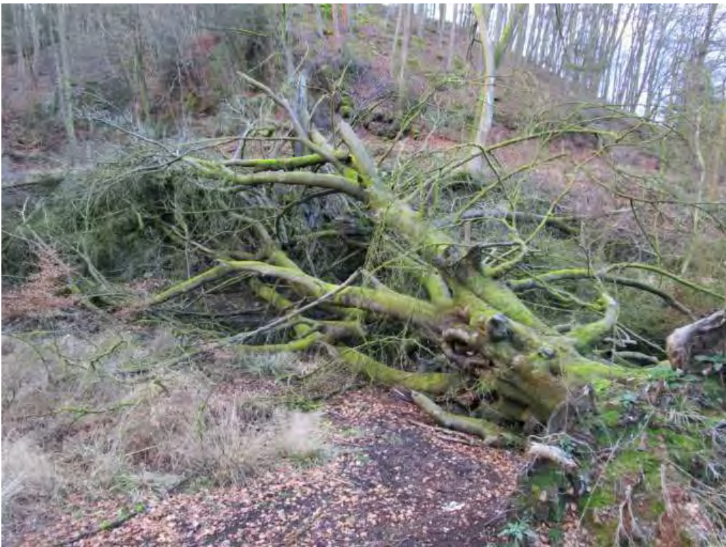
Recent Beech collapse onto stonework. Needs fairly urgent removal as restricting channel. Direction photographer facing:
