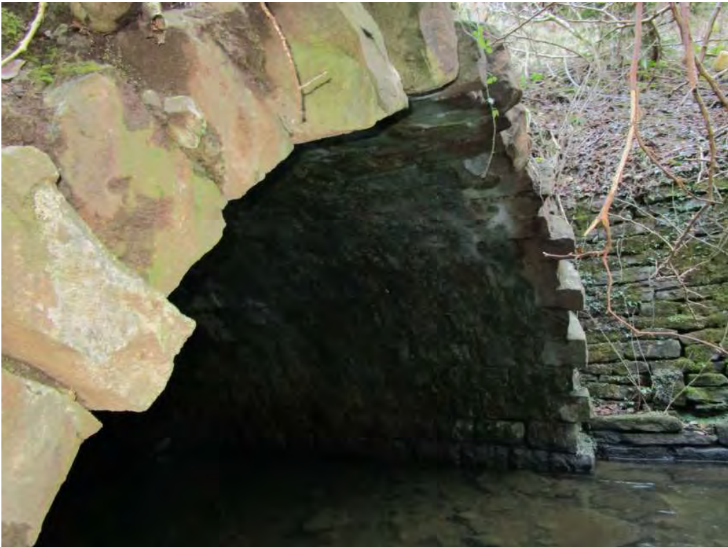
Tunnel entrance needing repair. Direction photographer facing: North East
