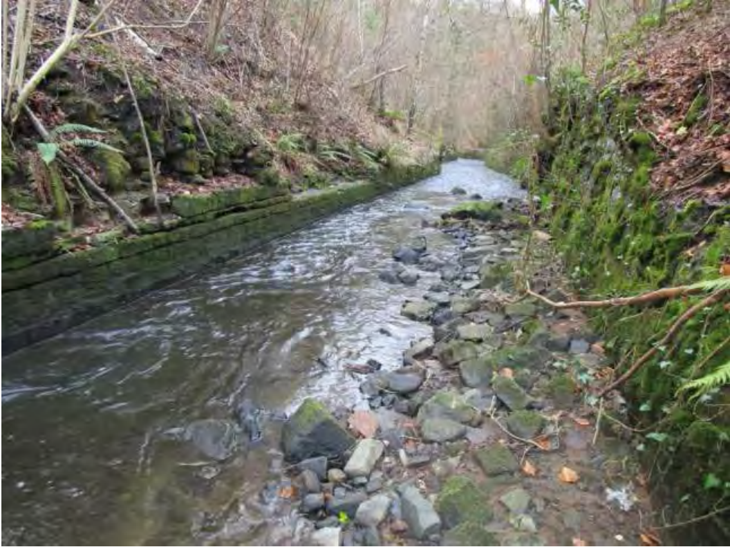
Stream bed needing stone removal and repointing. Direction photographer facing: South
