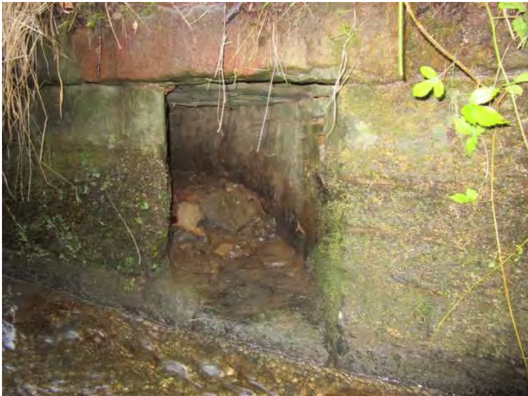
A stone inlet entering the main channel. Direction photographer facing: North East
