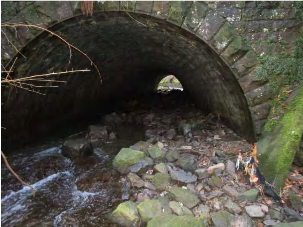
One of the three tunnels needing stone removal. Direction photographer facing: North
