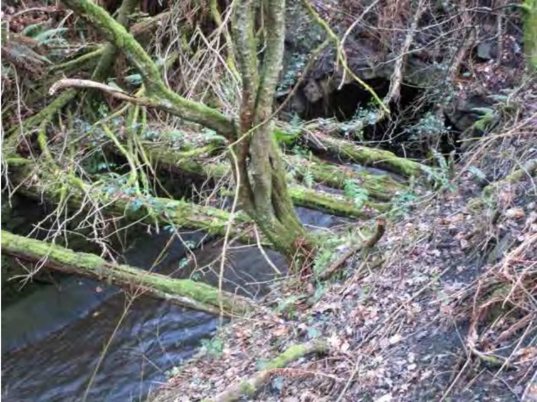
Stream bed continues via tunnel, under road to Ruspidge Direction photographer facing: North West
